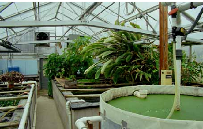
Ecological Engine Designed by John Todd Research and Design to Process Wastewater on Site
